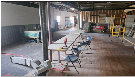
Photo by Glenn Miller Current condition of upstairs hall.
